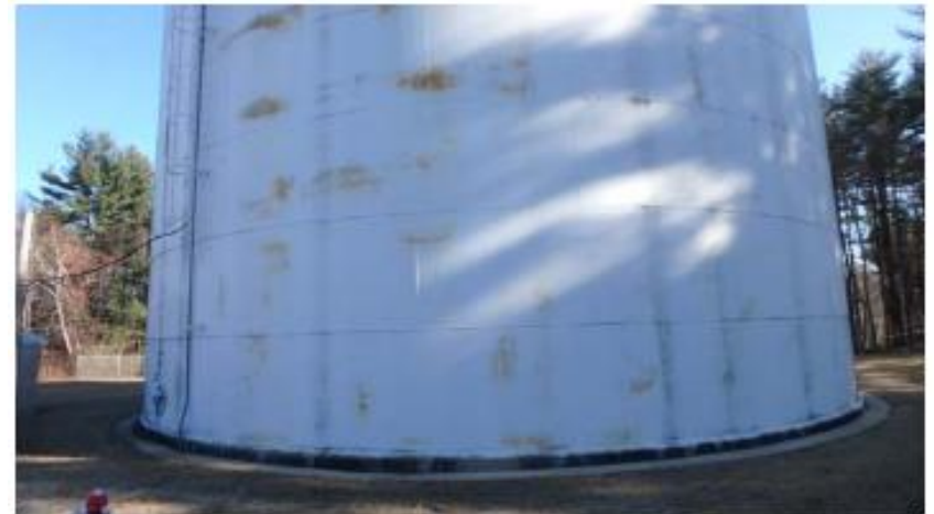
Coating degradation led to corrosion
